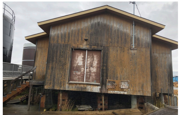
Foundation failure caused Nunapicuaq’s washeteria to temporarily close in 2022, leaving the village without running water for cleaning dishes, flushing toilets, and laundry. Photo: Susan Natali/Woodwell Climate Research Center.
